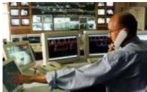
Integrated Control Systems
